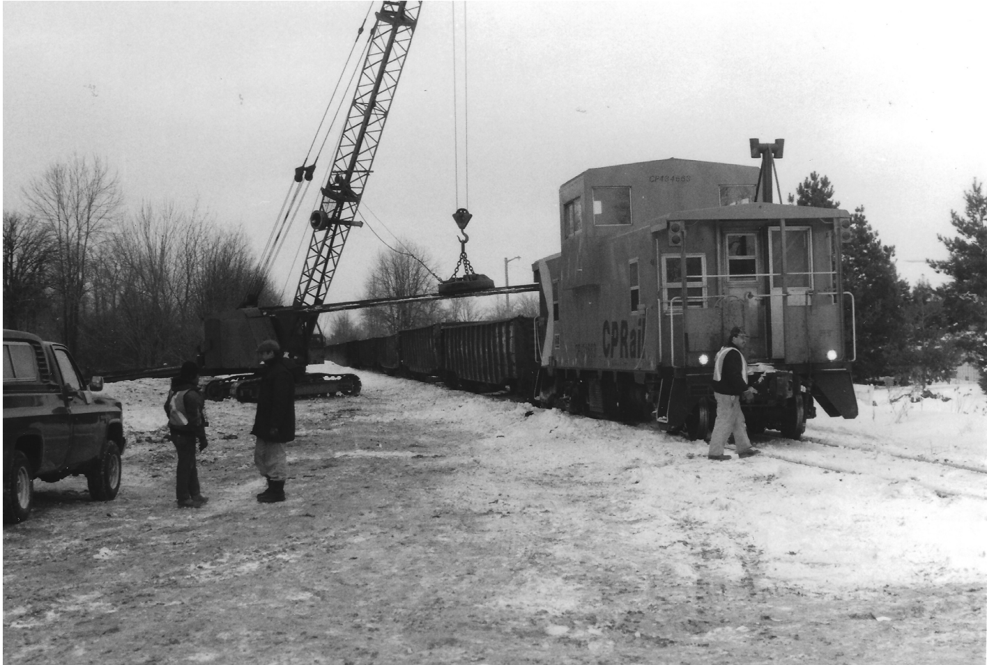
Bulldozers are clearing away the snow at the Verona Station site. The track lifting crew are getting equipment in place to continue the lifting of the rails.
