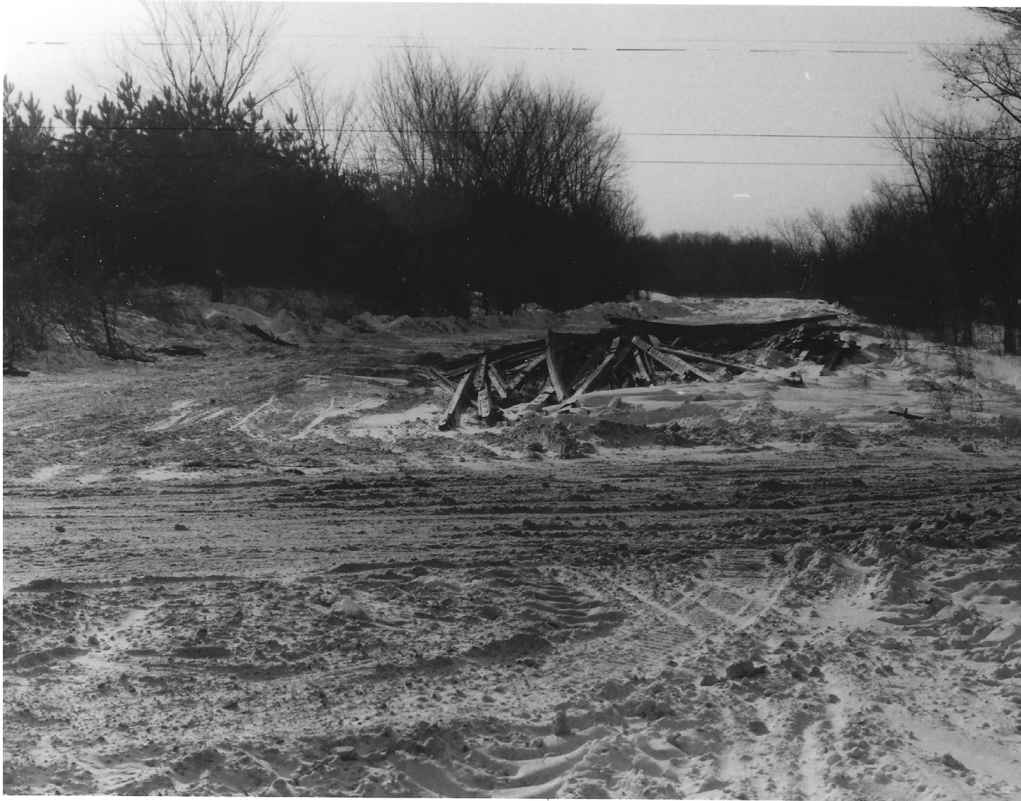
The rail line looking north toward the Murvale Station, from the Orser Road crossing. Mile Board 90 is on the pole at left. A crane truck and crawler tractor are parked at the crossing. Sections of rail are lying on the snow-covered ground.
