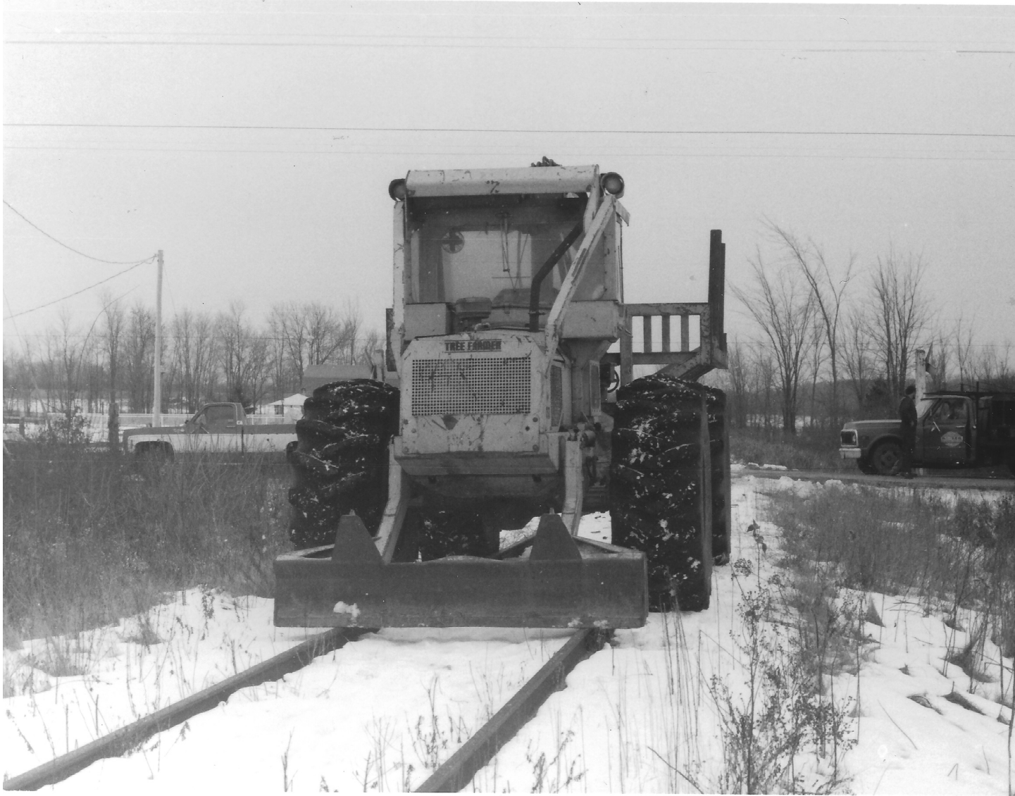
The rail line looking south from the Orser Road crossing. The pile of rails is to loaded onto trucks and hauled to Harrowsmith.
