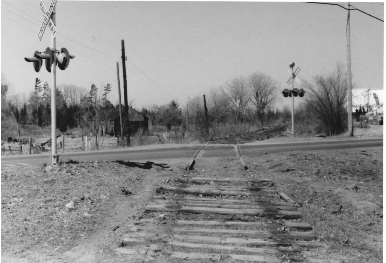
The rail line looking north upgrade toward the Sydenham Road crossing. The white electrical control box on the post at left is for the automatic signals at the road crossing.
