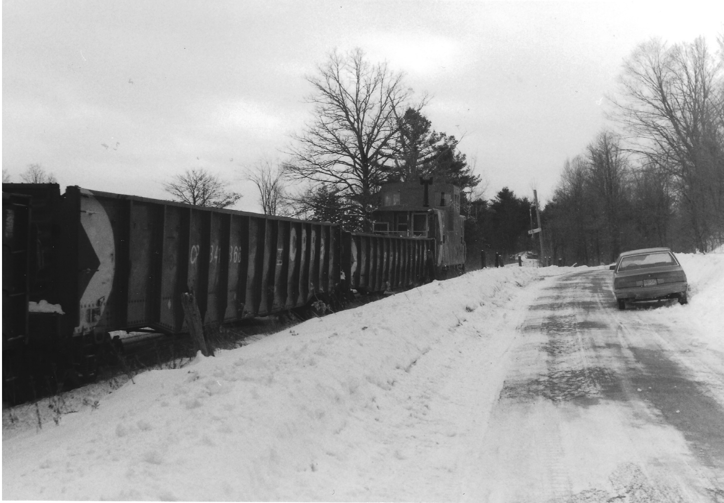
This CP Rail work train consisting two locomotives, thirteen gondola cars, and a caboose at the Verona Station site. The train is facing north. Loading of the rails is almost completed.
