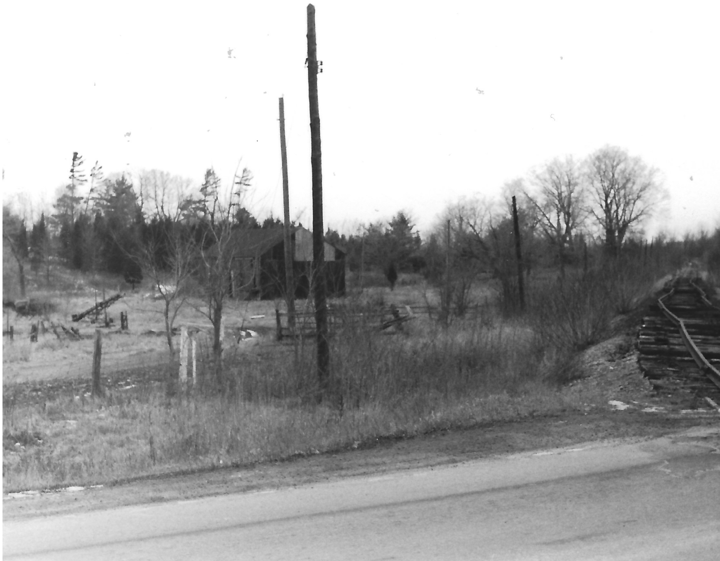
The Sydenham Road crossing, looking south, showing both rails lifted two days earlier. Both rails were lifted by [a] rail lifting machine simultaneously.
