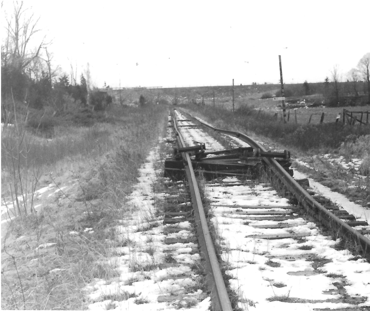
The crawler tractor with the track lifting machine [was left] when the work was stopped for the New Year period.
