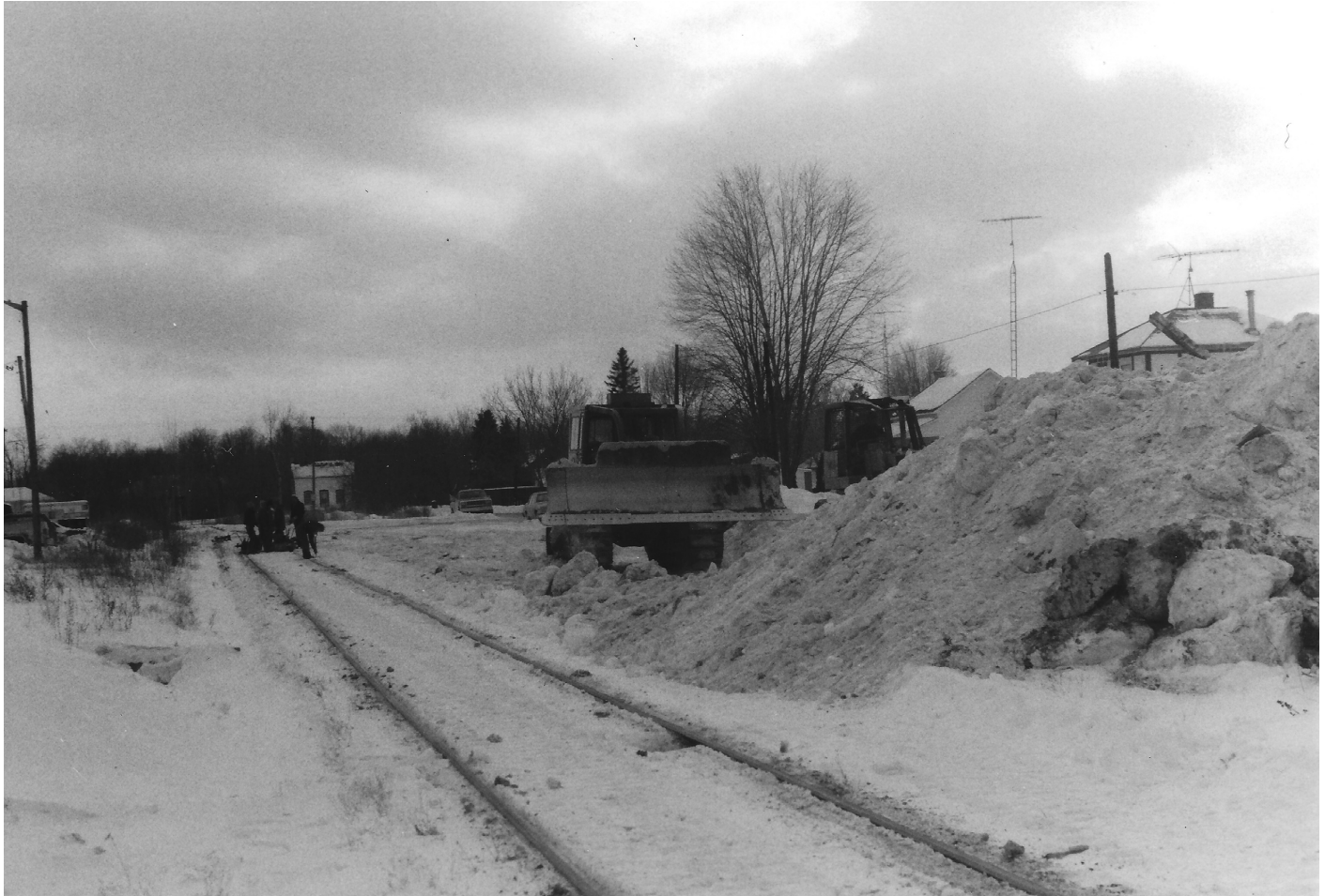
A track crew, behind the caboose, is using a rail machine to remove the nuts from the bolts at the rail joints. The track lifting steel sleds in the foreground are pulled by a bulldozer to lift the rails from the ties. The west (left) rail has been lifted. The view is looking north.
