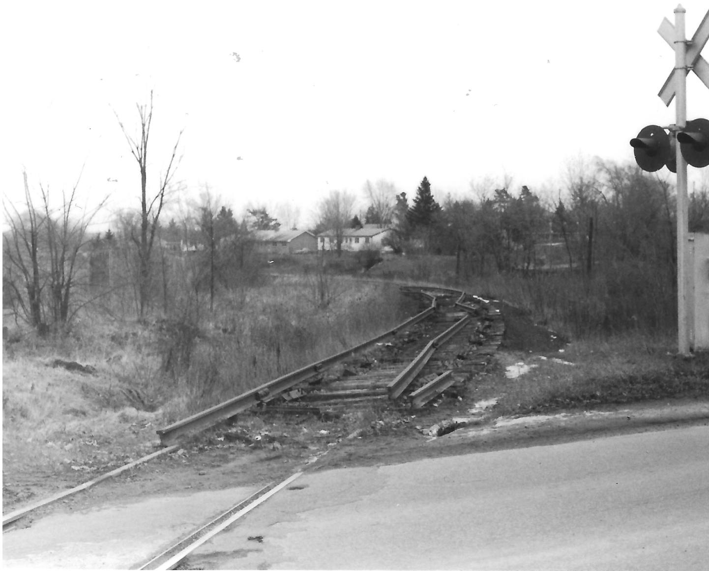
The rail line at Mile 97 looking south from the McIvor Road Crossing. The track lifting machine was left in this position over the New Years. Hwy 401 overpass is in the background [ you can see milepost 97 on the right].
