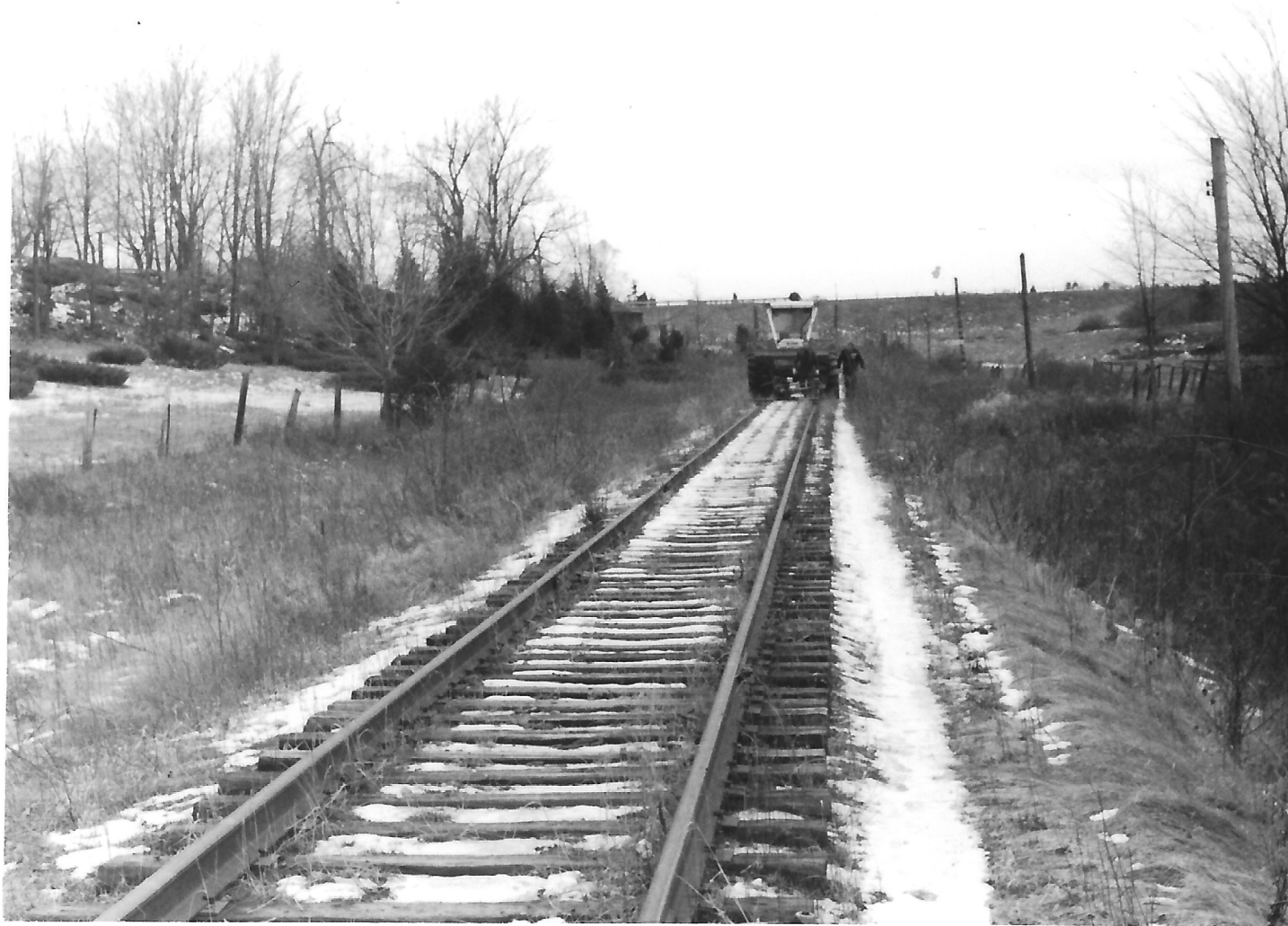
The rail line looking north at the McIvor Road crossing. Photo taken in late morning. In the afternoon, the rails were lifted from the Sydenham crossing to Mile 97 just south of the crossing. The rail machine is used to remove nuts at the rail joints.
