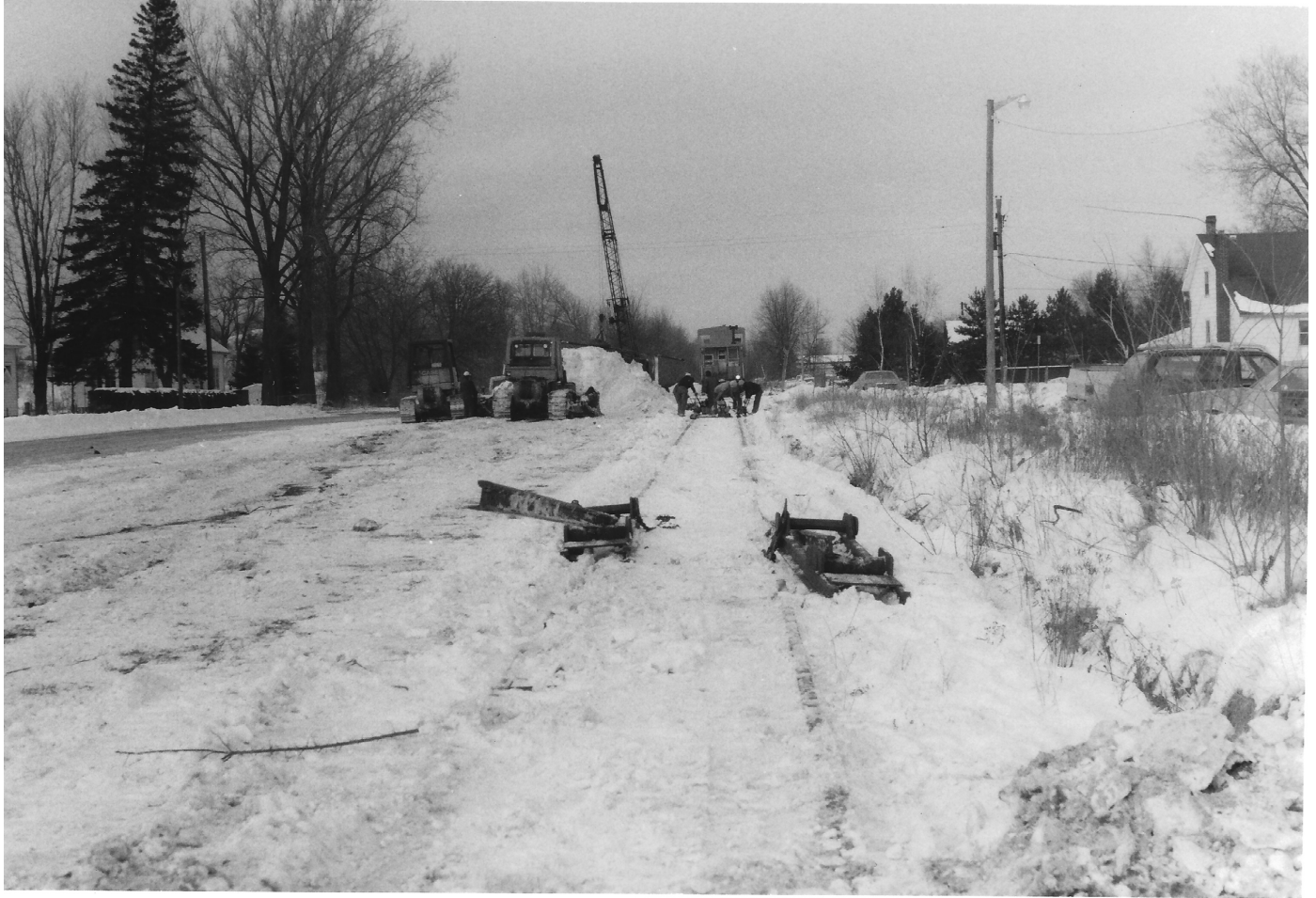
The CP Rail work train ... entering the Craig Road crossing north of Verona. The cars have been loaded with the track rail at Verona. This was the last train to operate over the rail line. The rails on this line were lifted two days later.
