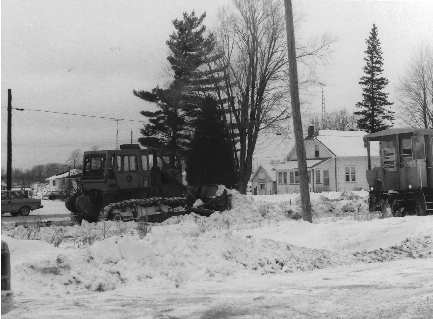
This CP Rail work train of thirteen gondola cars, loaded with track rail at Verona is approach the Old Frontenac Road crossing south of Godfrey, at Mile Board 75. This was the last train to operate over the rail line. The rails on this line were lifted two days later.
